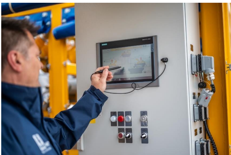
(2) The complete plant can be operated from a single screen in master-slave mode. All images: © BAUER Group
